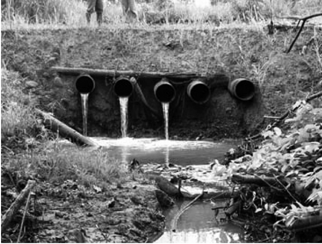
The discharge pipes.
